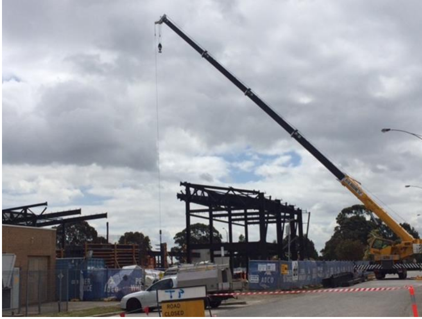
Construction works underway for the new Trades Centre at Morwell campus due for completion in 2021
